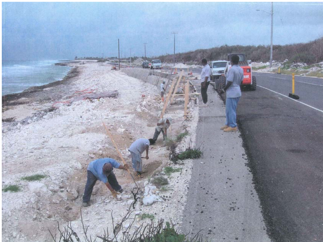
October 2005 – NRA crew working on 400ft long sea wall at Clarinda Beach
