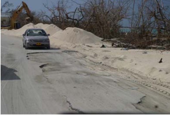
With Hurricane Ivan storm surge removed part of the asphalt on West Bay Road north of Public Beach.
