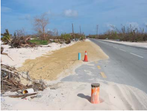
North of the Marriot Courtyard – October 5, 2004. NRA facilitated road clearance and temporary patch
