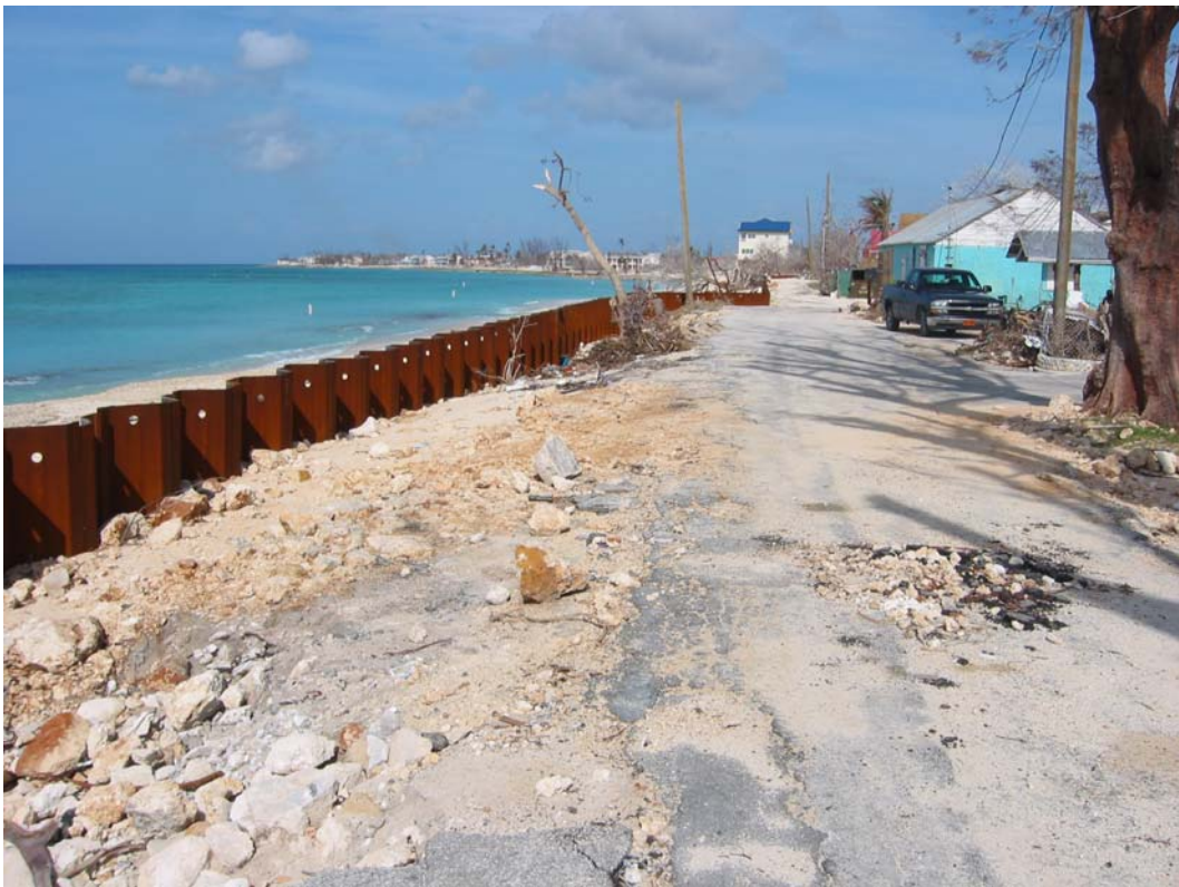
Boggy Sand Road - washout
